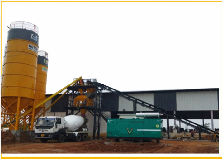
Inline Bin, Conveyor - Conveyor System with Waiting Hopper
